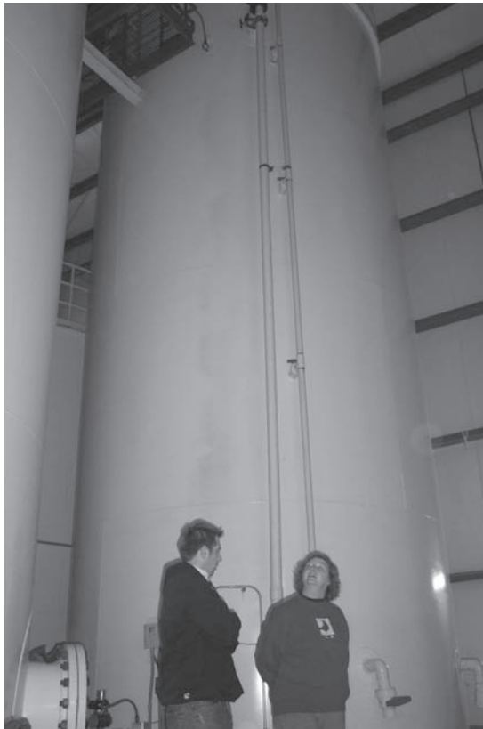
Fig. 23.2 IBR anaerobic digester.
